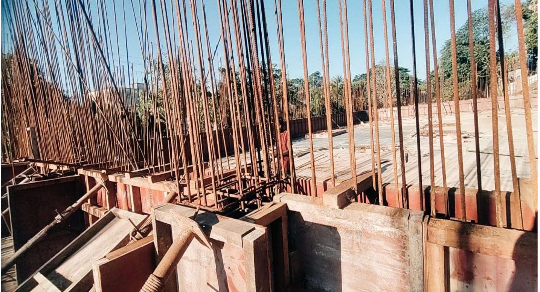
15 MLD STP at Abhoynagar, Agartala
