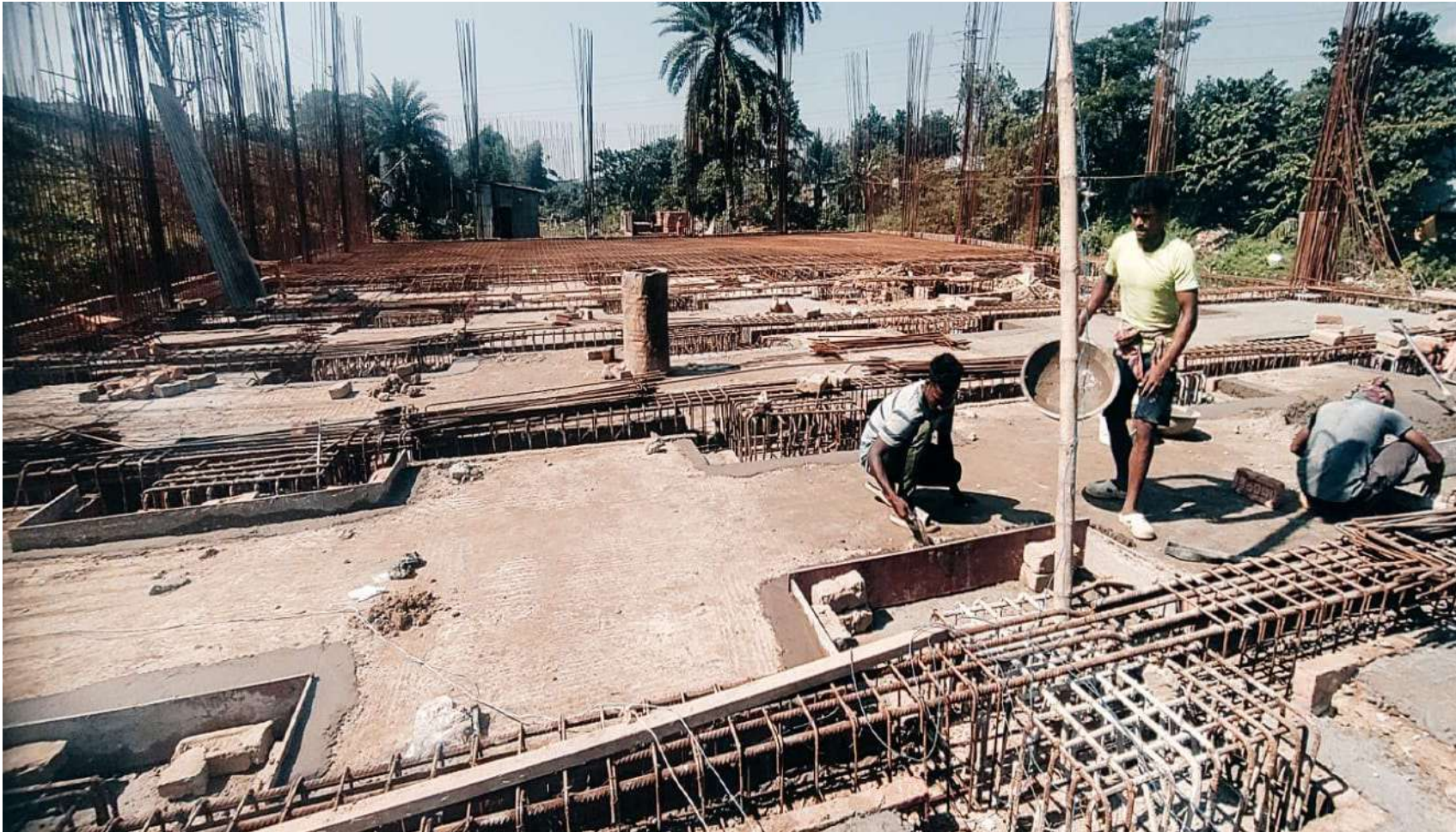
15 MLD STP at Abhoynagar, Agartala
