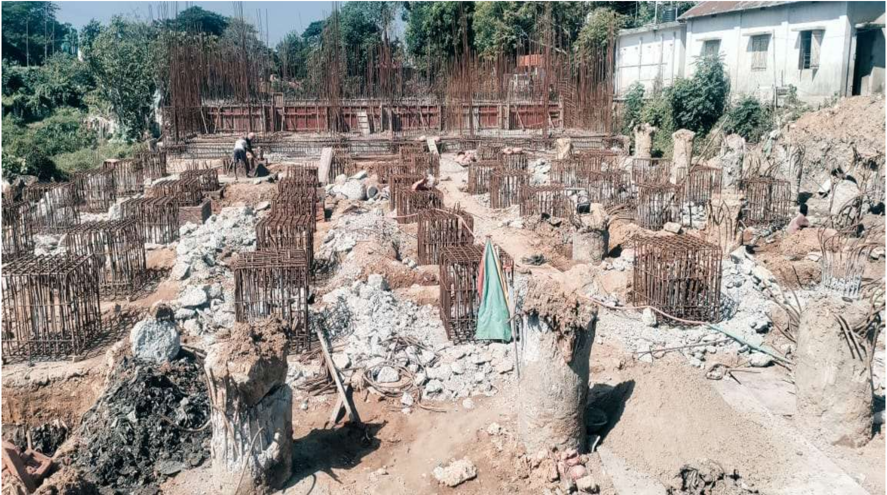
10 MLD STP at Ranjitnagar, Agartala
